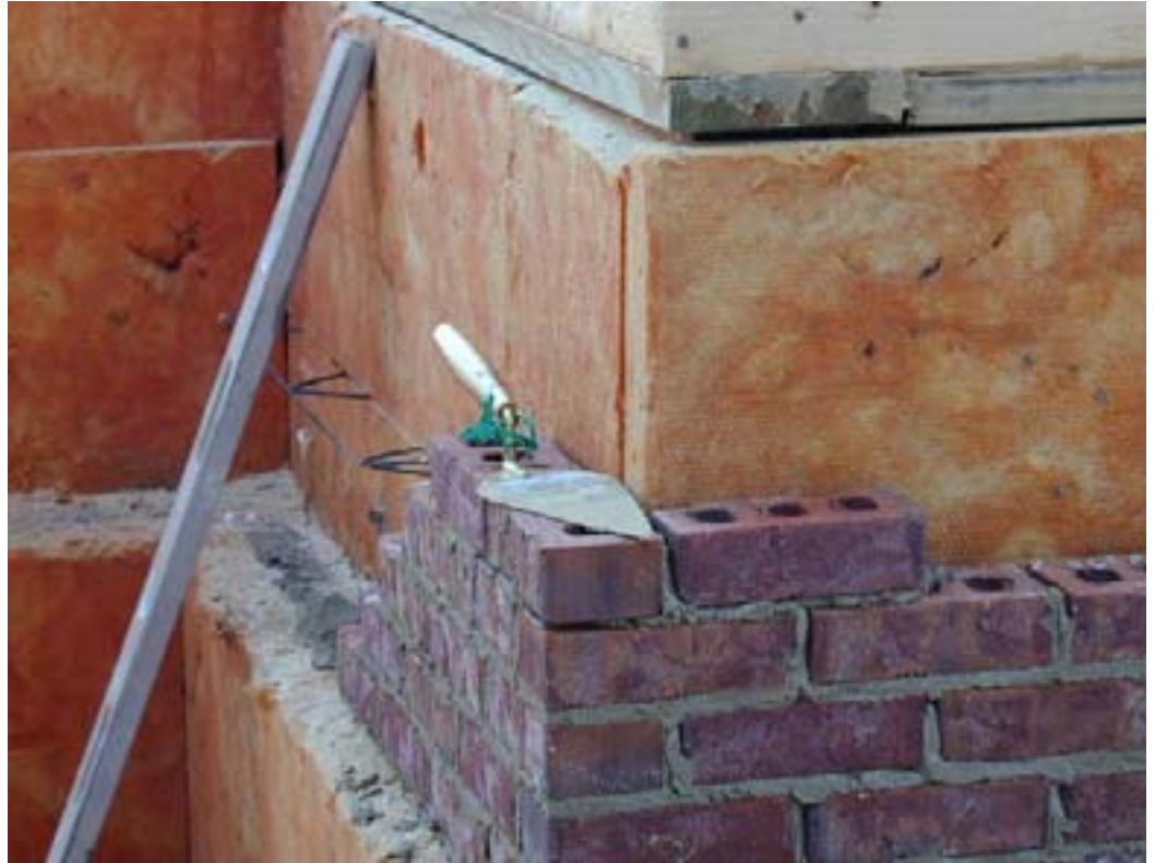
Figure 5. Insulation of foundations below grade at Estate Homes. Brick ledge is created by stepping from a 12 in. block to 6 in. block
